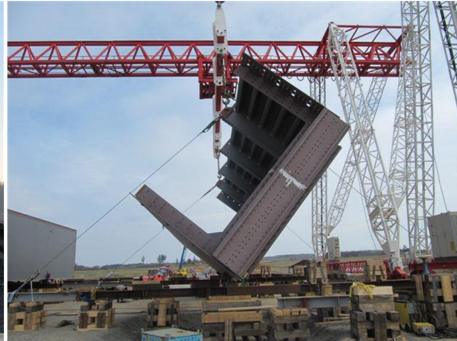
Erection of preassembled side walls with parts of bottom and orthotropic plate
